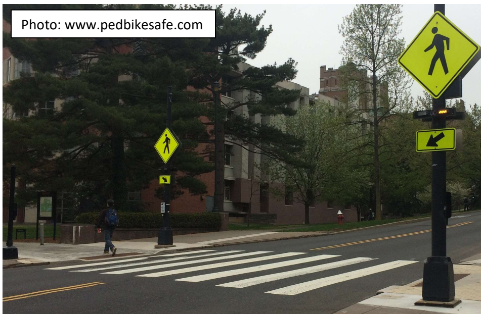
Figure 3 – Sample of High-visibility crosswalk and and pedestrian activated warning lights suggested for Monocacy Way trail crossing at Schoenersville Rd (CAT concept)
